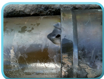
A Leak in Plastic Piping
