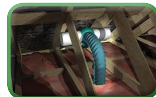
Attic Installation Setup
